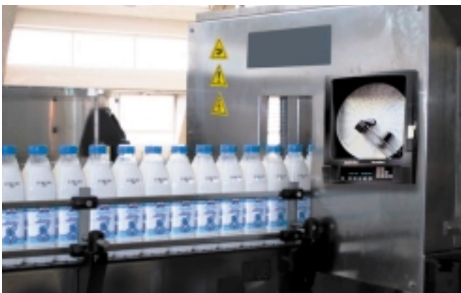
Typical Application – Bottling Line
